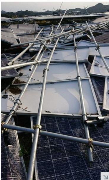
Damage to solar panels caused by 2019's 15th typhoon is seen in Chiba Prefecture in this file photo from October that year. (Mainichi)
